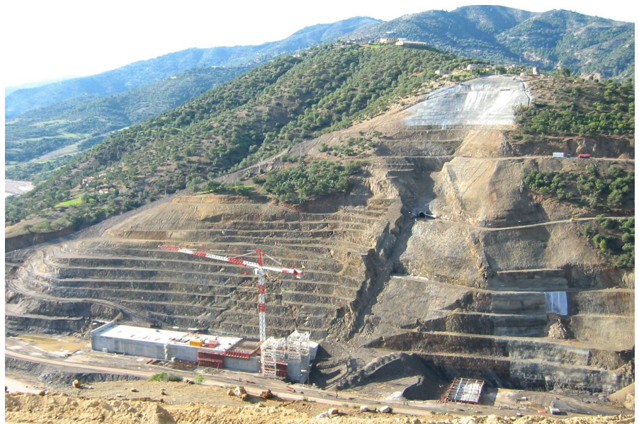
Movements and landslides threaten the workers ad the stability of the dam
