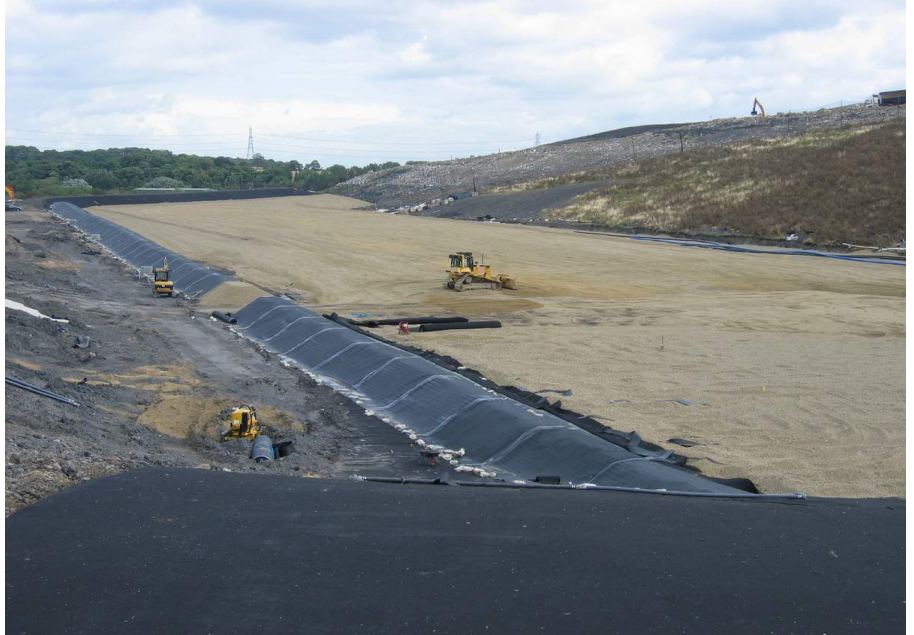
Top left : Installation of settlement cells within foundation trench. Top right : Reservoir enclosure for each settlement cell. Bottom : Welbeck instrumented cell.
