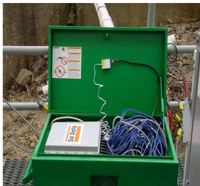
Datalogger connected by phonenumber communication to a central computer
