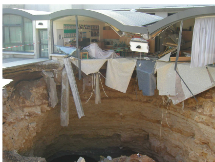
The schoolyard collapse
