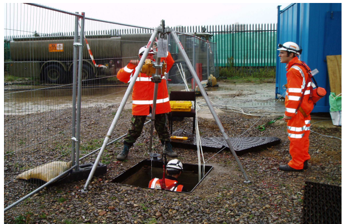
ABOVE: Confined space installation team enter the tunnel with a tripod and fall arrestor.
