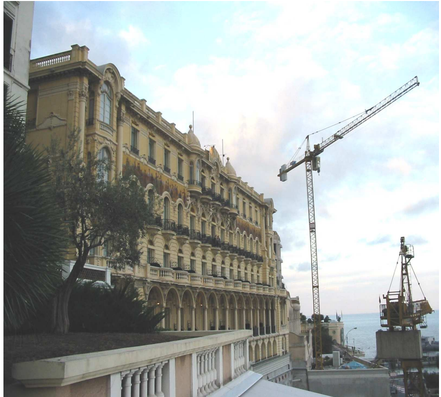
Facade of the Hermitage Hotel. 16 tri-axial sensors were installed on the key structural elements of the building
